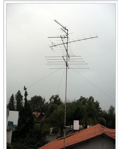
Rooftop television antennas. Yagi-Uda antennas like these six are widely used at VHF and UHF frequencies.
